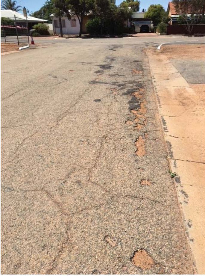
Above: Memorial Ave requiring patching and sealing
