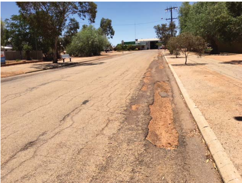
Above: Maddock Street requires patching and edge sealing
